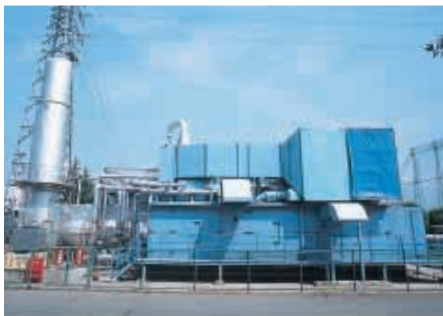
Co-generation plant (Kofu Factory)
