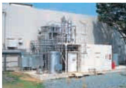
Dichloromethane recovery plant (Kofu Factory)
