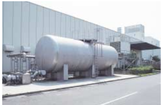
Industrial water reuse plant (Kofu Factory)
