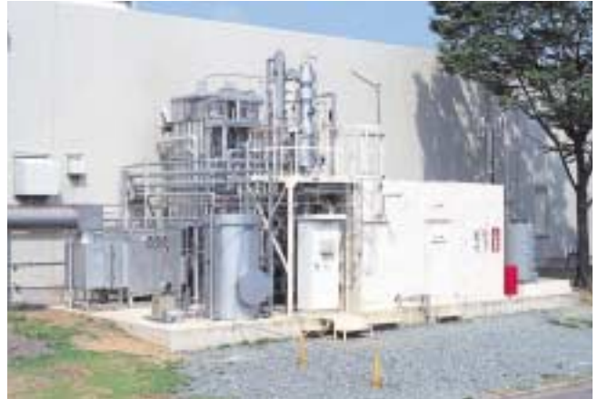
Dichloromethane recovery plant (Kofu Factory)
