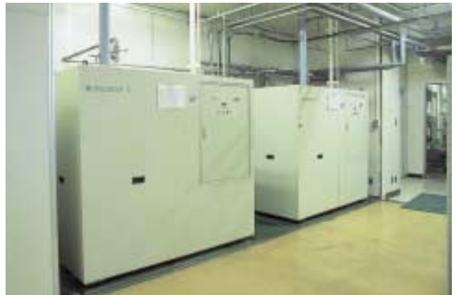
Dichloromethane recovery plant (Ashitaka Factory)
