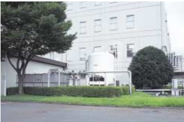
Industrial water reuse plant (Fujinomiya Factory)
