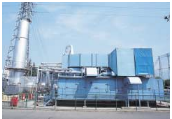
Co-generation plant (Kofu Factory)
