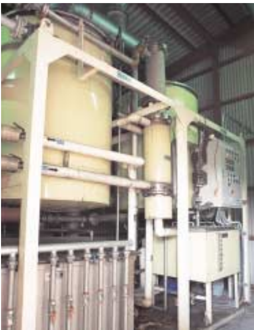
Equipment for recovering ozone-depleting substances (Ashitaka Factory)
